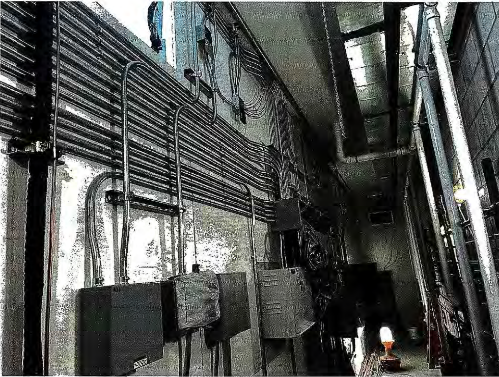
Westbound Hardin Rest Area – Mechanical Room (Dick Anderson Construction/Tyler Hansen)
