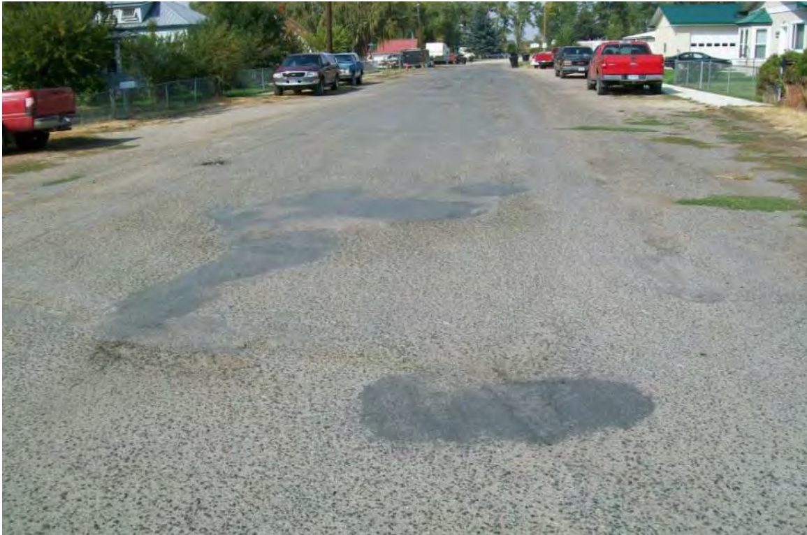
Maryland Ave. at Clark St. PASER-4
