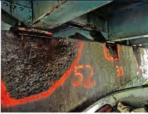
Pictured above: The pre-repair condition of the bridge's concrete cap shows the loss of support under the girder bearings.
