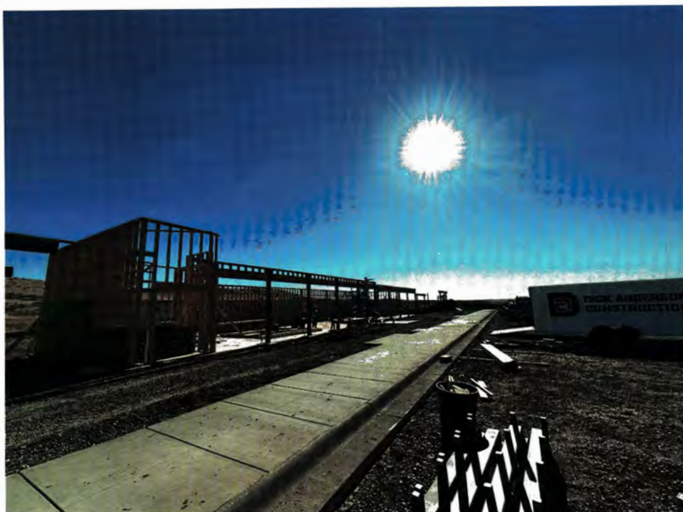
Interior walls of main building being constructed at the westbound site of the Hardin Rest Area (Dick Anderson Construction/Tyler Hansen)
