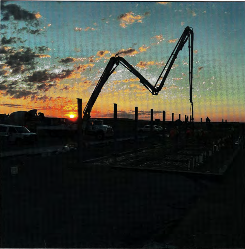
Concrete boom pump truck installing the concrete slab for the main building at the eastbound rest area site. (Dick Anderson Construction/Tyler Hansen)
